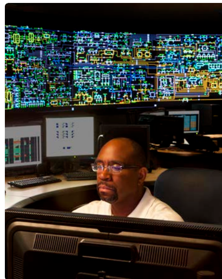
At PECO's Transmission Operations center in Philadelphia, operators keep close watch on the regional electric grid. PECO serves 1.6 million electric customers and nearly 500,000 natural gas customers.
