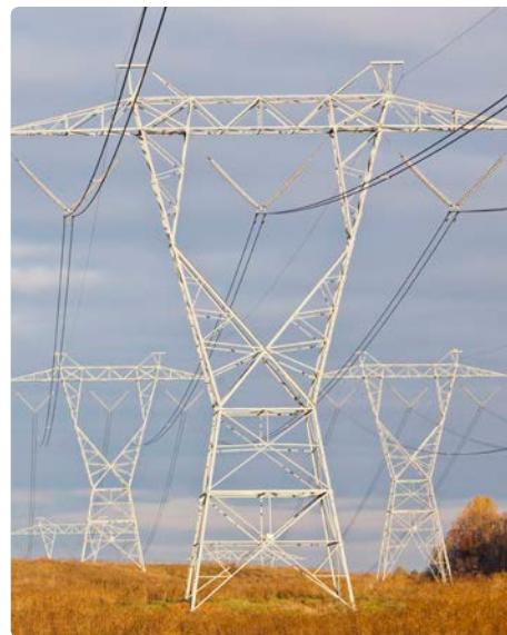
ComEd laid the groundwork for the Grand Prairie Gateway, a major transmission infrastructure investment projected to save customers approximately $500 million by reducing system congestion and driving cleaner energy to the grid.
